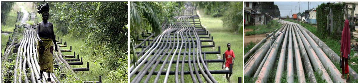
Exposed easily accessed and difficult to secure Oil Pipelines in the Niger Delta (Ibeleke, 2016 / Akinleye, 2016 / Faul, 2016)
