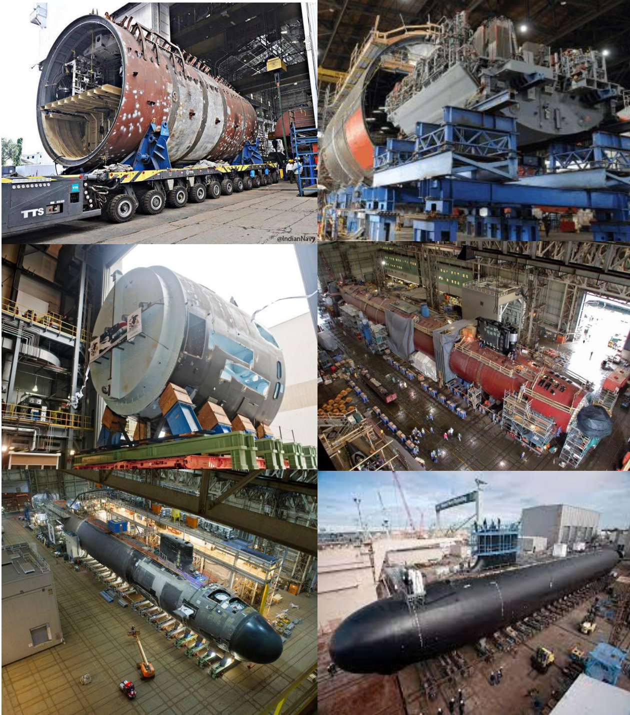
Figure 67: Modular construction of modern submarine 283 (Virginia-class nuclear power submarine of the US Navy) 284
