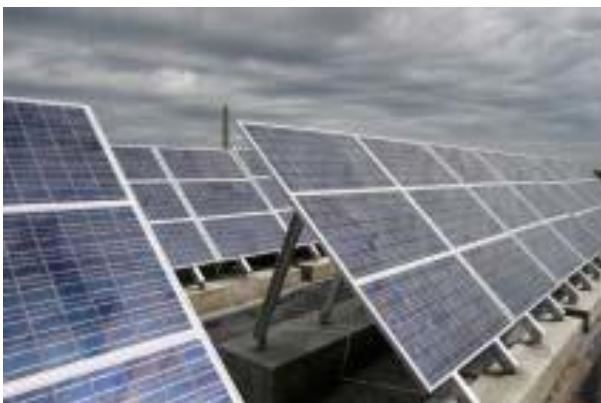
PV installation on roof. (Amogpai, A ,2011)
