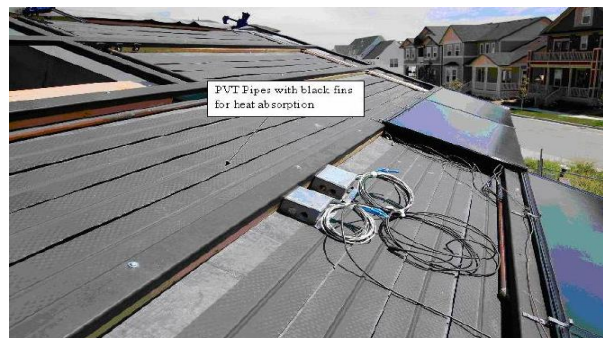
Figure 11: PVT system with pipes and fins on the University of Colorado 2007 Solar Decathlon house Source: (Horizon Renewals, 2013)
