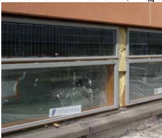
Figure 16: Window integrated PV installation.
