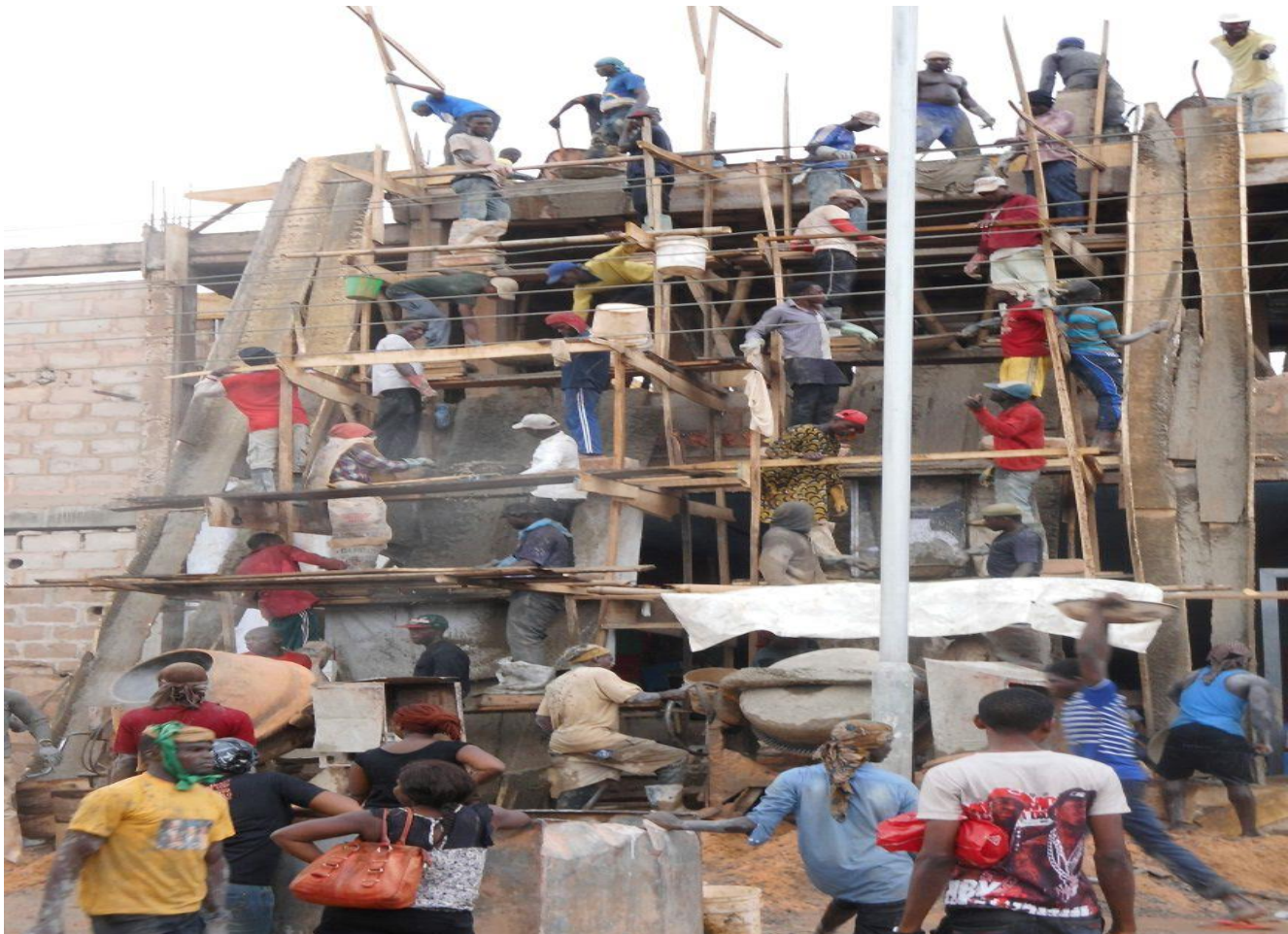
Picture 4: Construction workers at work; producing and transporting concrete onto the deck of a building.
